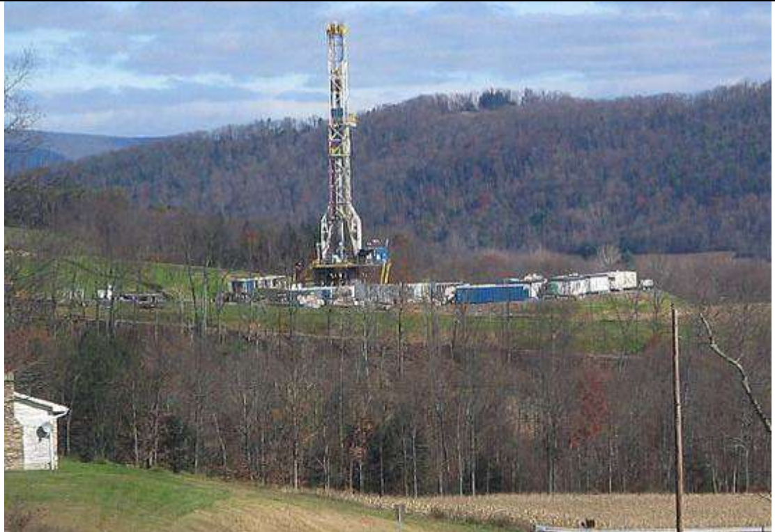
Photo: This is what hydraulic fracturing towers look like. The photo shows a platform set for drilling into the Marcellus Shale Formation for natural gas in Pennsylvania. Credit: Ruhrfisch
