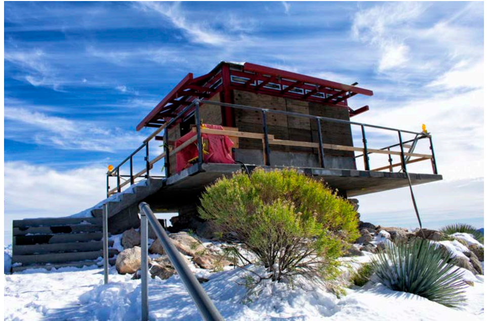
Vetter Lookout December 3, 2019 - On a snow hike to Vetter Mt., we got a close up look at the progress on reconstruction of the lookout using fire resistant materials—steel and concrete. Photos: https://www.flickr.com/photos/cscurlock/albums/72157712047948677
