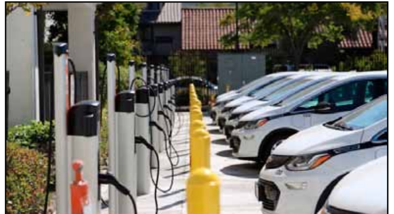
Santa Barbara MTD recently installed 14 new ChargePoint Level 2 electric vehicle chargers for a new fleet of all-electric light duty vehicles of 14 2020 Chevy Bolts. The new fleet replaces aging gasoline-powered sedans. SoCal Edison covered the costs of upgrades and the SB APCD provided significant grant funds. (photo contributed)
