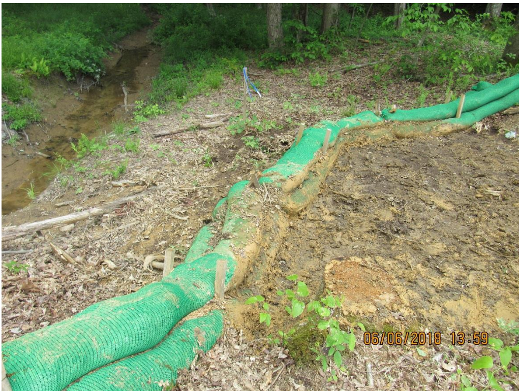
Photo 2: Station 6782+00 control failure repair but additional controls not added.
