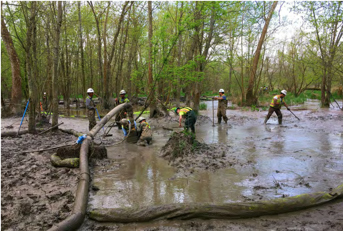
Cleanup effort of the Rover Pipeline spill in Stark County, Ohio
