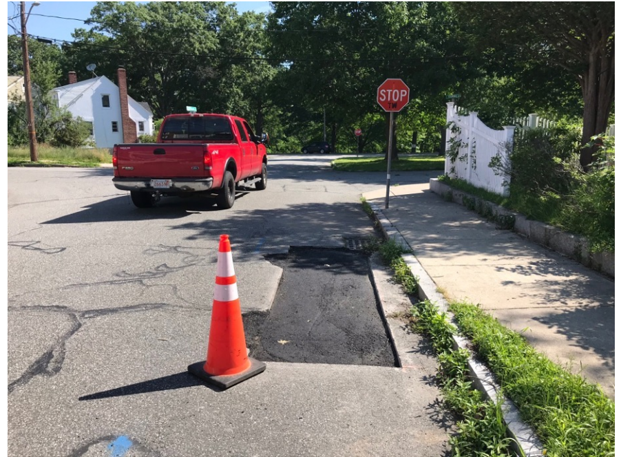
Infiltration trench in Arlington, MA
