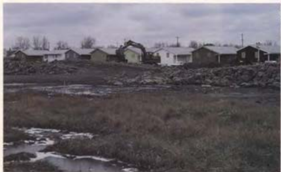
In these backyards forever: The Love Canal landfill is not part of the EPA's "final" cleanup.
