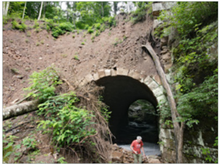
Same Culvert After a Landslide PHOTO: STEPHEN STROTHERS.
