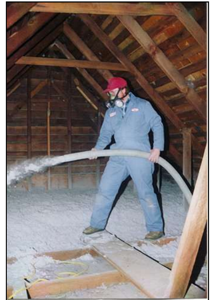
Insulation being applied to a building. Photo credit: National Renewable Energy Laboratory
