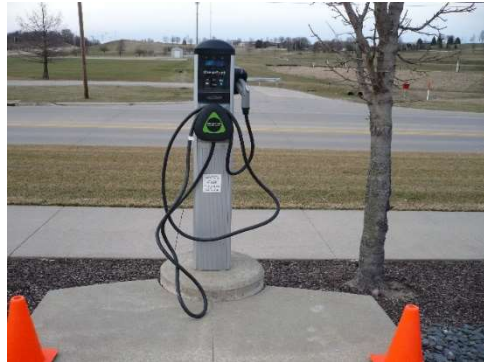
Charging station at Kirkwood Community College. Photo by Pam Mackey Taylor
