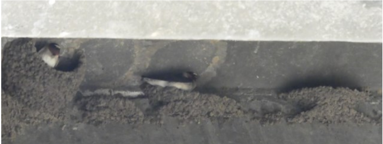
Nesting activity under the Laurel Street Bridge in the areas identified in the first photo.
