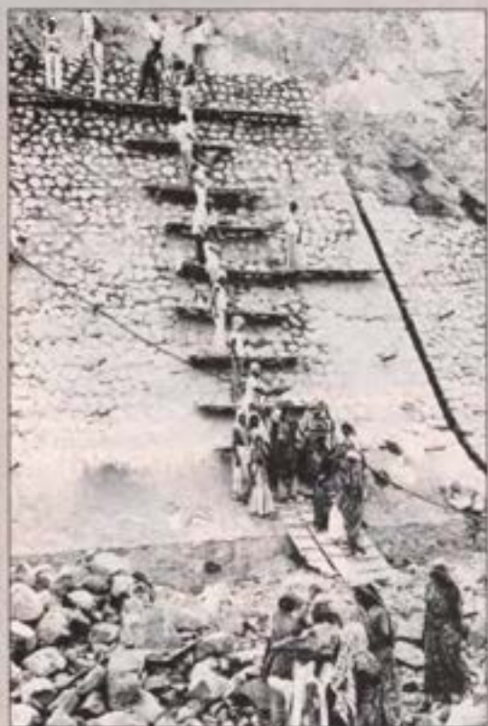
Local laborers, who make up the project's nontechnical workforce, use stones to line one of the hundreds of irrigation channels.
