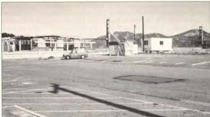
Construction of the Presidio post office was well under way when a judge declared it illegal. The decision is an important victory for both San Francisco and the national park system.
