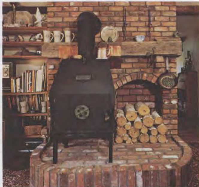
Wood-burning stove in the family room supplements the house's passive solar system. In the winters since the house was built, temperatures have been maintained at a comfortable 70°, using heat captured by the solar system and by burning wood gathered by owners.
