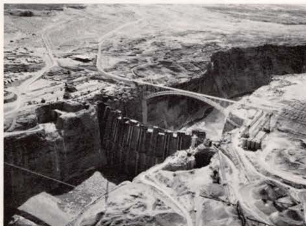
Glen Canyon dam and bridge in northern Arizona (just below the Utah-Arizona boundary line) as it looked from the air on April 7, 1963. When completed in 1964, it will rise 580 feet above the river bed to a crest elevation of 3715 feet. Photo by Bruce M. Kilgore
