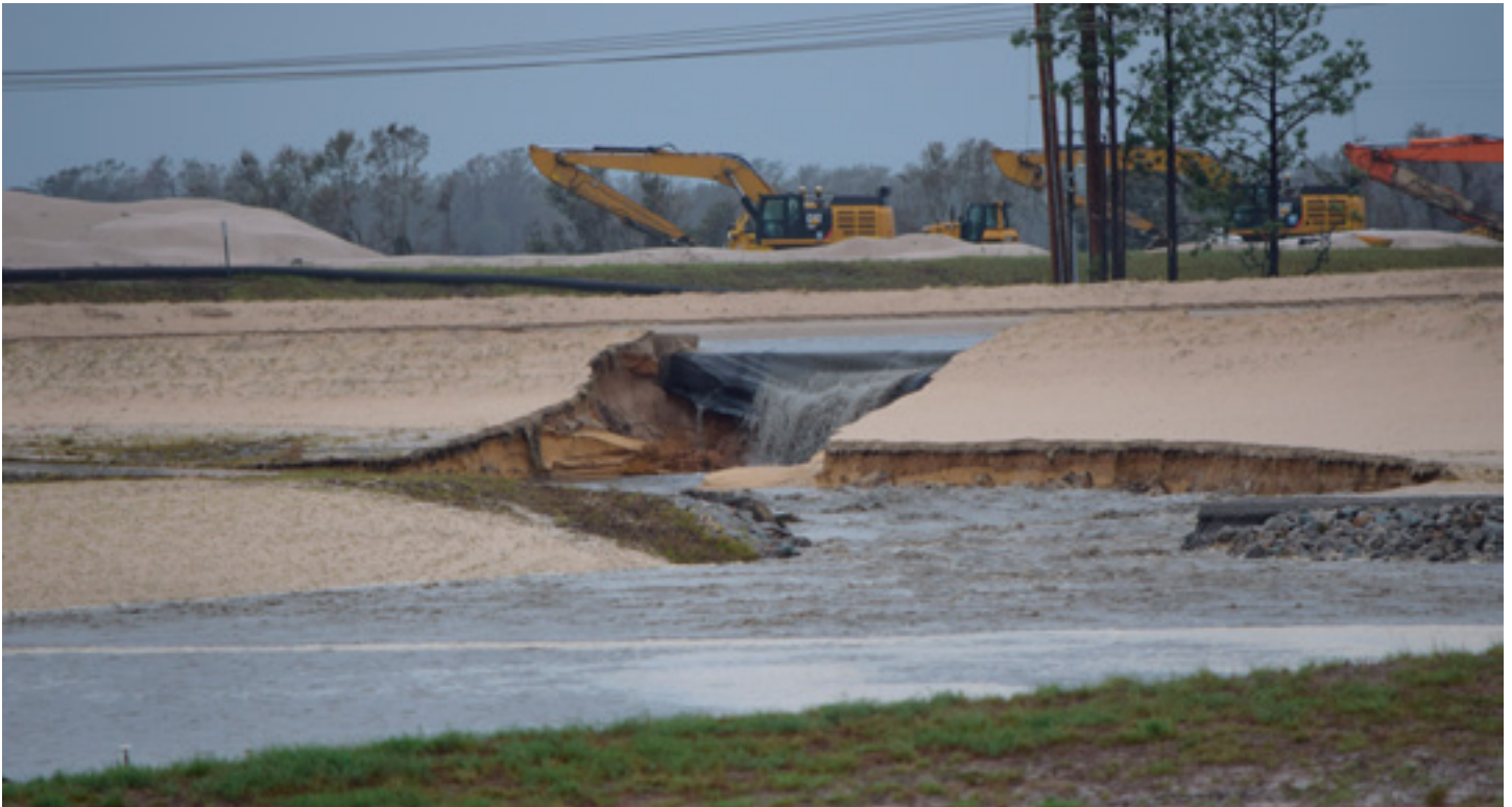
COAL ASH SPILL AT THE L.V. SUTTON POWER STATION OUTSIDE WILMINGTON, NC. PHOTO: CAPE FEAR RIVERKEEPER
