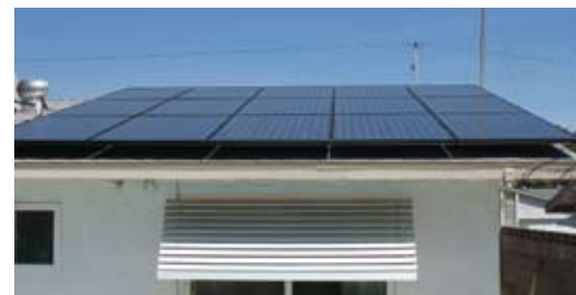
PV on roof. Photo: Steve Rypka.
