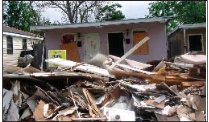
Demolition debris in the lower ninth ward. (4/07)
