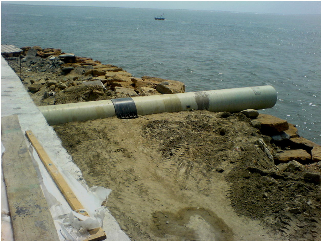
Brine outfall pipe at desalination plant. Photo by Tafasir Khichi.
