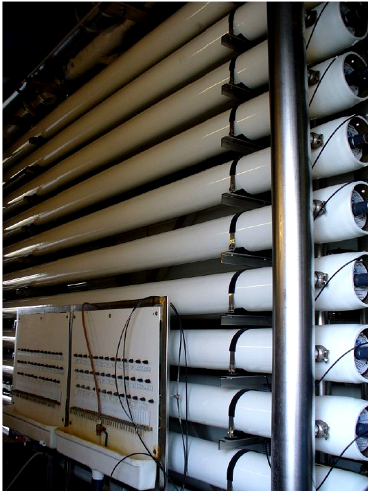
Racks of high pressure filter tubes at Lower RioGrande plant. Photo by Texas Water Resources Institute
