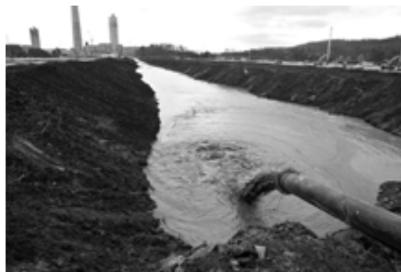
Ash and water discharge into holding area at the Tennessee Valley Authority's Kingston Fossil Plant during the cleanup phase in March 2009. Source: TVA
